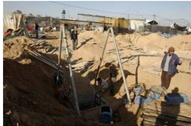
Repairing a tunnel damaged during Operation Cast Lead (Hamas's PALDF Forum, January 24, 2009).
