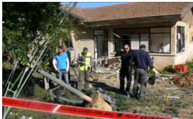
House in Sderot hit by a Qassam rocket (Photo by Meital Ohayon, www.sderotmedia.com , February 26, 2009).
