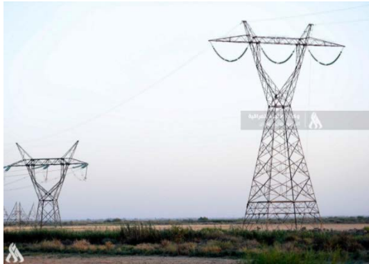
High-voltage pylons in Iraq (Iraqi News Agency, August 17, 2021)
