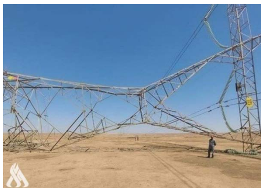
High-voltage pylon sabotaged by ISIS (Iraqi News Agency, August 16, 2021)
