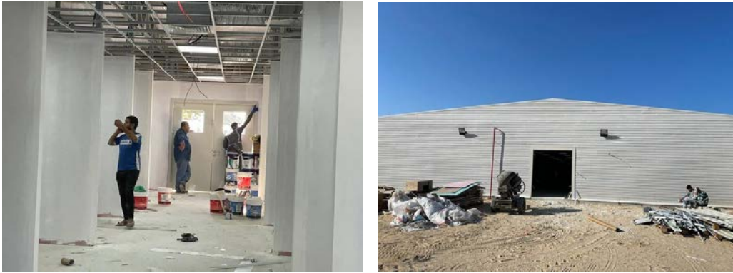
Despite the decline in coronavirus infection, construction continues for a new UAE-funded field hospital for coronavirus patients near the European Hospital in eastern Khan Yunis (Safa Facebook page, October 21, 2021).
